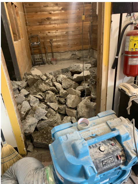
- the old concrete pad under the bathrooms being demolished to install new plumbing for main floor access from the theatre foyer - WITHOUT STEPS!
